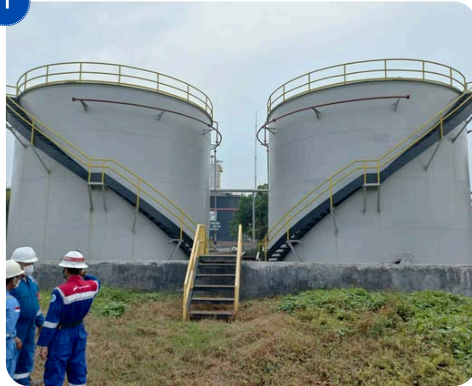
Tank and Flaring System Repair in SP Cilamaya Utara Subang Field PT PERTAMINA EP Zona 7
