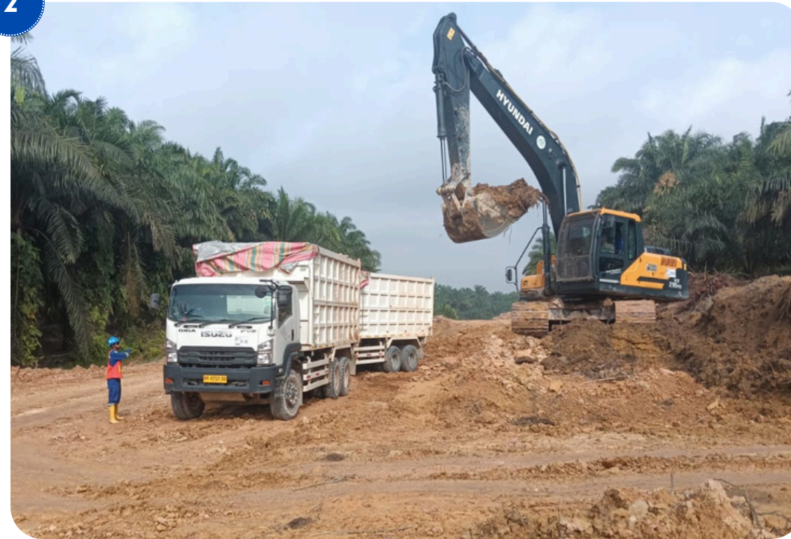
CONSTRUCTION SERVICES WORK UNIT RATE EARTHWORK SOUTH AREA (CS WUR EW SA)-PAKET 4 PGAS SOLUTION DI WK ROKAN PERTAMINA HULU ROKAN (PHR)
